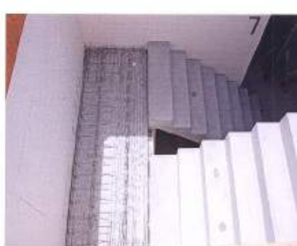
Emfil Stair fixed on Emfil landing
